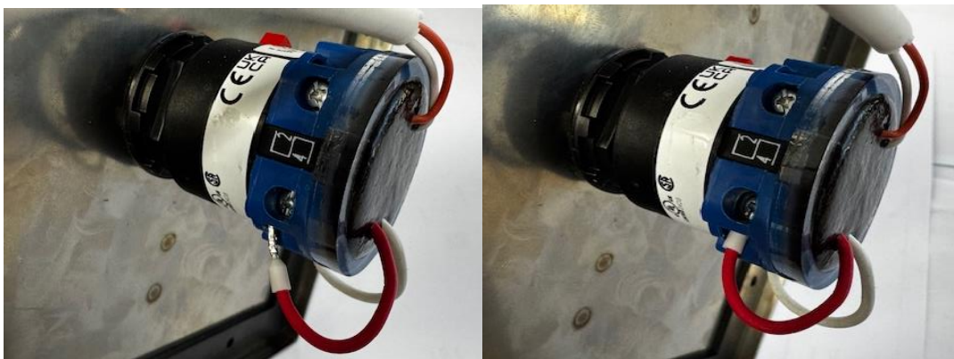
Figure 3. Example of loose vs correctly secured wires
