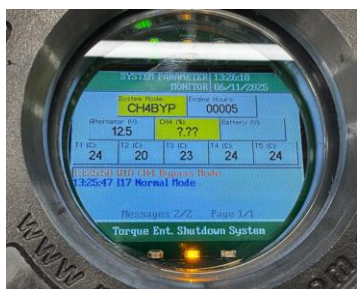
Figure 1. CH 4 Bypass Mode shown on the screen.
